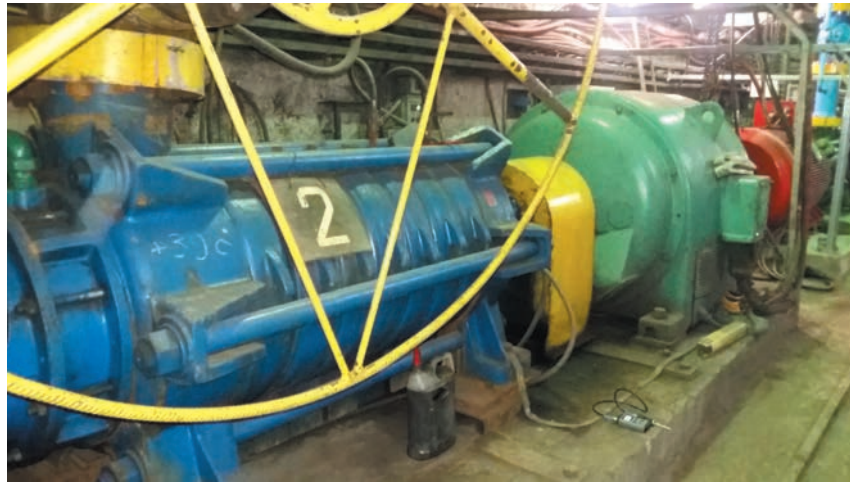
Fig. 2. Pump unit no. 2
