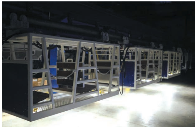
Fig. 4. Mobile lighting of passenger stations from the CA-190 battery-powered suspended locomotive (white light – the locomotive is at the passenger station)
