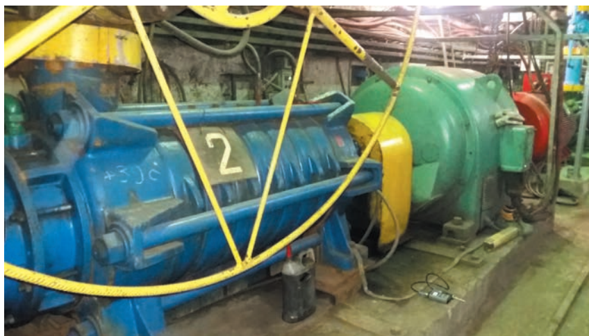
Fig. 2. Pomp unit no. 2
